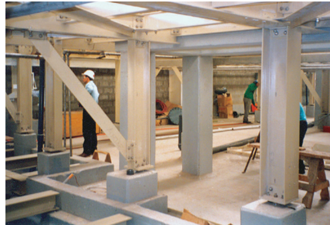
EXTREN® structural shapes were used in a SXEW copper refinery because of the highly corrosive environment.
