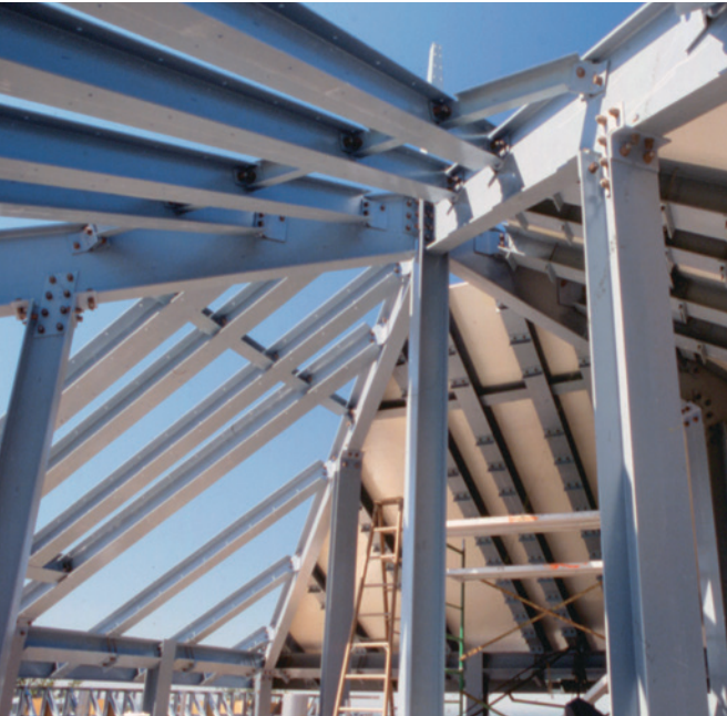
This entire rooftop structure was built using EXTREN®, to take advantage of its transparency to RF and cellular signals.
